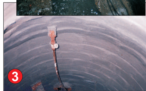
3. The result - protected, sealed and waterproofed - ENECRETE® WS has sealed and protected in a few easy steps.
