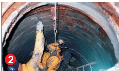
2. After active leaks have been plugged with ENECRETE® WP, the walls are brushed with two coats of WS - the water sealer.
