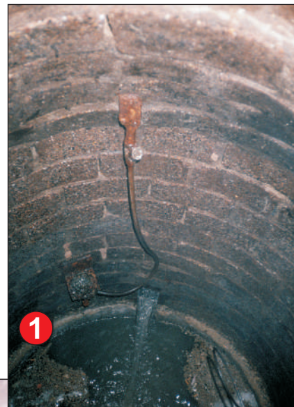
1. The problem - walls under chemical attack with active water leaks...
